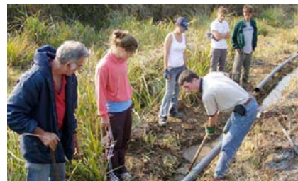
Team members work together as they prepare for installation of a ram pump system in KwaZulu-Natal, South Africa.
